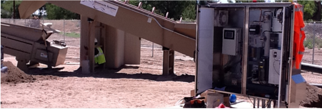
Figure 5. Electronic control panel with sand washer in background.
