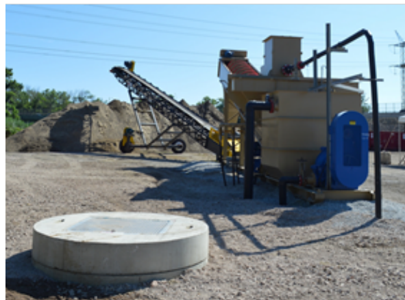
Figure 9. Cuyahoga River shore-based plant with concrete access port to pump wet well in foreground.
