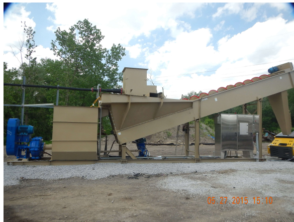
Figure 10. Skid-mounted sand washer with scalping box, overflow sump, injection water pump, and control panel.
