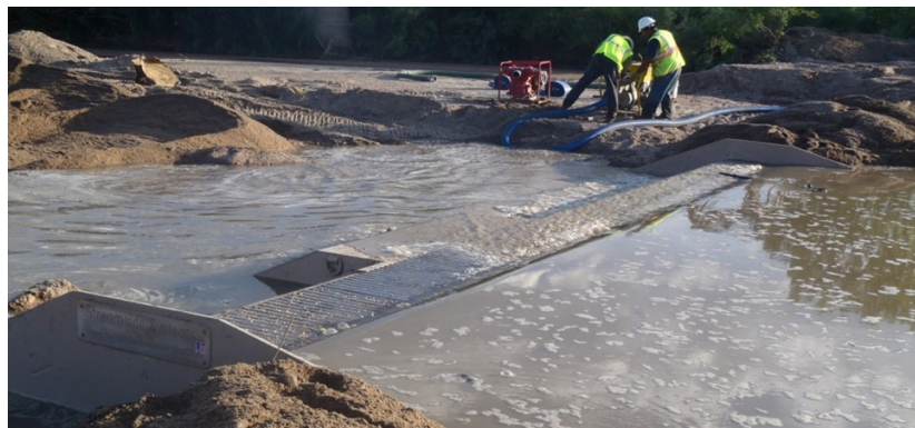
Figure 2. Bedload Collector installed at Fountain Creek.
