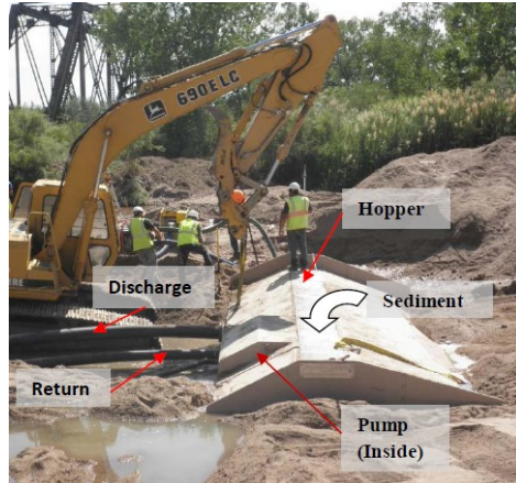
Figure 3. Bedload Collector components.
